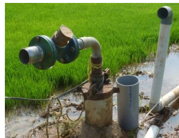
Flow meter installed on borewell
